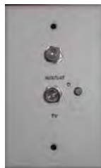
Antenna Power Supply
